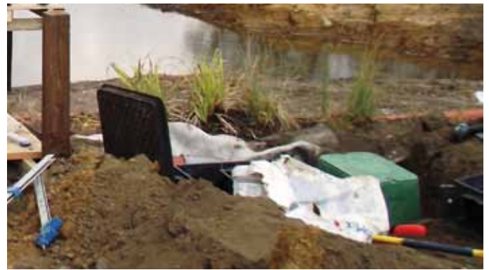
An auto water feed control system was situated within a pond side manhole. This unit will maintain the ponds mean water level when natural water loss occurs.
