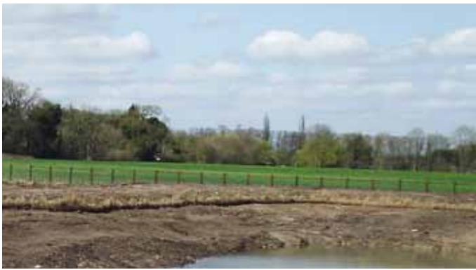
An edge detail of vegetated coir rolls were placed and secured around the ponds perimeter prior to flooding, this was followed by spot planting of aquatic species, including lilies, selected to establish in the pond.
